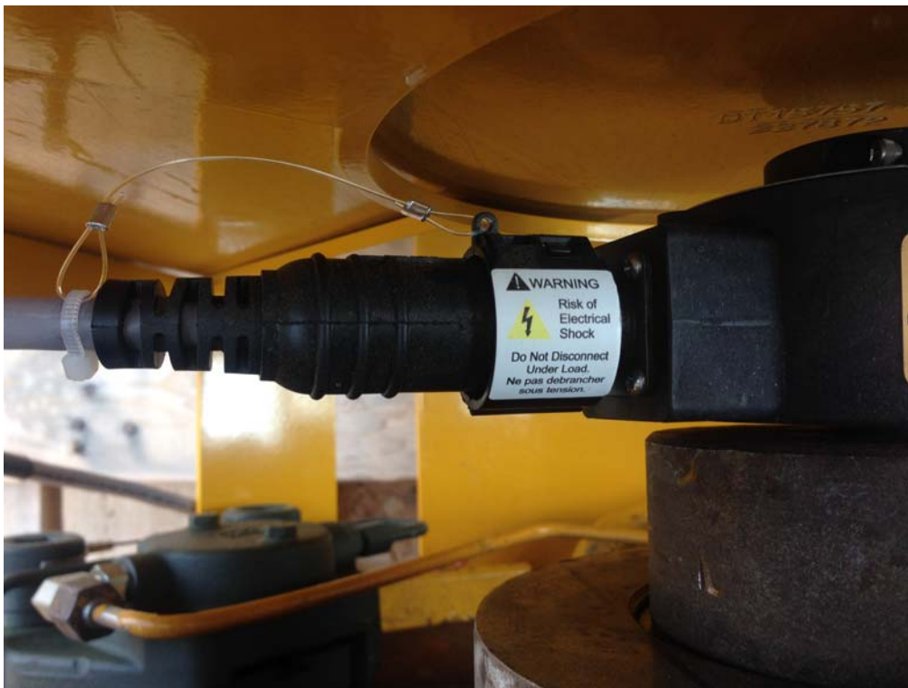
Figure 3: Encoder cable with lockout clip installed.
